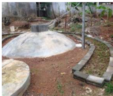
Biogas Digester at Boys Town –Diyagala
